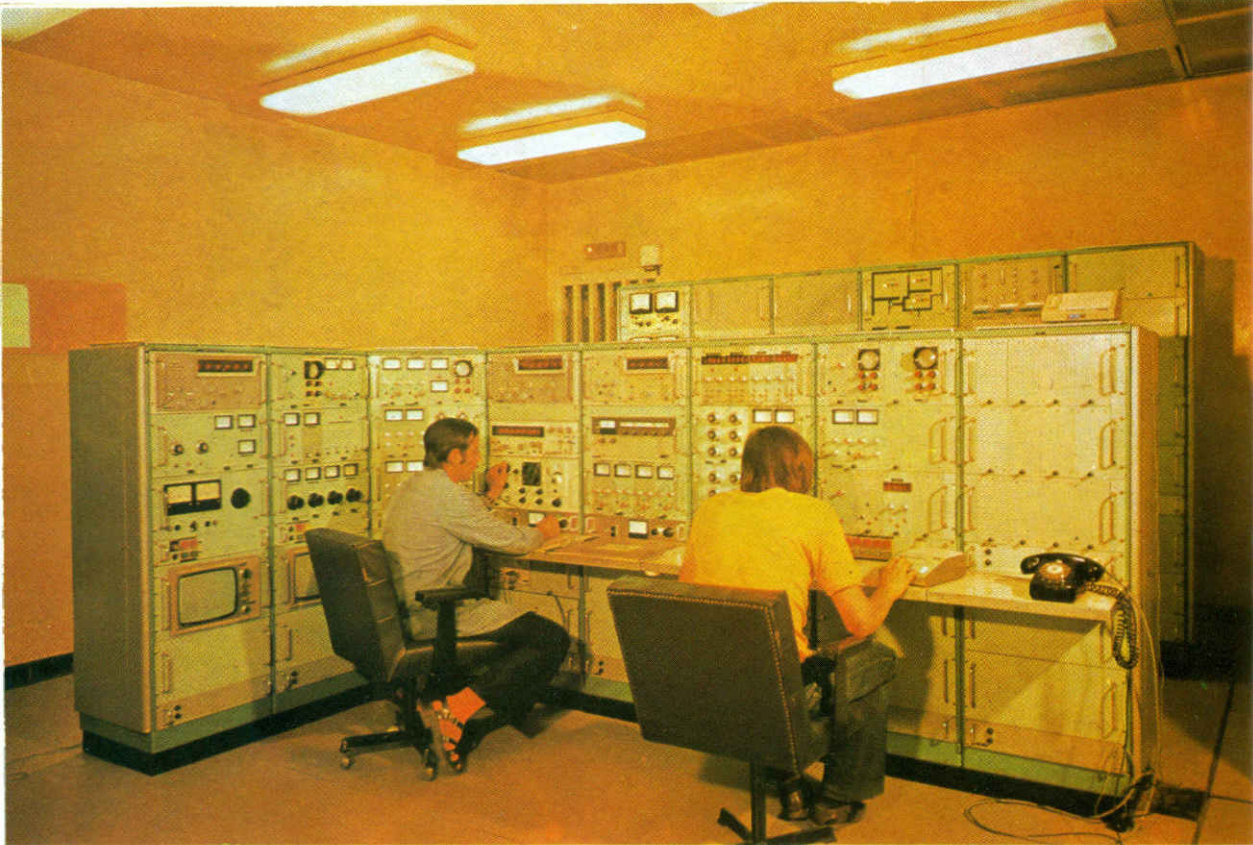
Control desk of the 5 MV Van de Graaff generator
